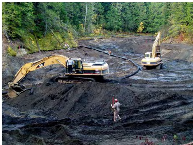
Figure 24. Mechanical excavation was used to remove 20,000 CY of sediment from this impoundment. Streamflow is routed through the black pipe to dewater the site completely (photo Inter-Fluve).
