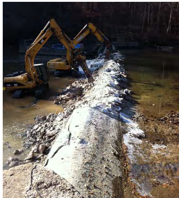
Figure 23. Jackhammers comb through a rebar reinforced concrete spillway during dam demolition (photo Inter-Fluve).
