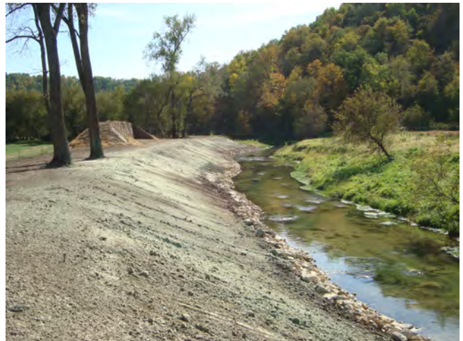
Fig. 11. Vertical nesting bank in background. Note its location set back from the stream channel.
