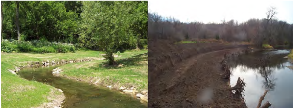
Fig. 15. Examples of two broad approaches to enhancing or restoring stream habitat. The figure on the left is a more traditional approach that uses a lot of rock to stabilize a stream channel and provide fish habitat (note the substantial amount of rock on both sides of the stream). The figure on the right represents a natural channel design approach that constructs a stable stream channel using geomorphology principles. Some natural channel design projects use woody debris, in addition to limited amounts of rock, for channel stabilization and fish cover (note the presence of root wads along the left bank in the photograph).
