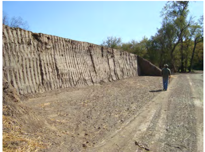
Fig. 10. Recently completed vertical nesting bank constructed as part of a stream restoration project.
