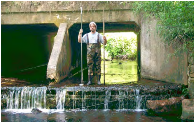
Fig. 14. Perched culverts, such as this culvert on Trout Brook in Dakota County, Minnesota, may prohibit trout movements during most stream flow conditions, except large floods. Credit: D. Dieterman.
