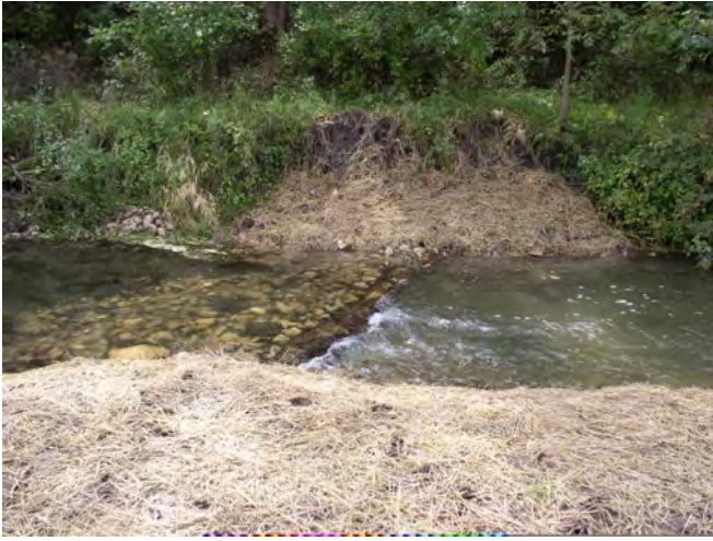
Fig. 13. Crosslog used to create pool habitat as part of a stream restoration project.
